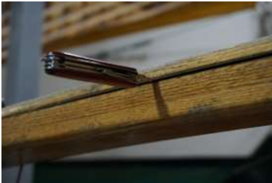
Figure 10.19 Bowsprit laminate compromised
