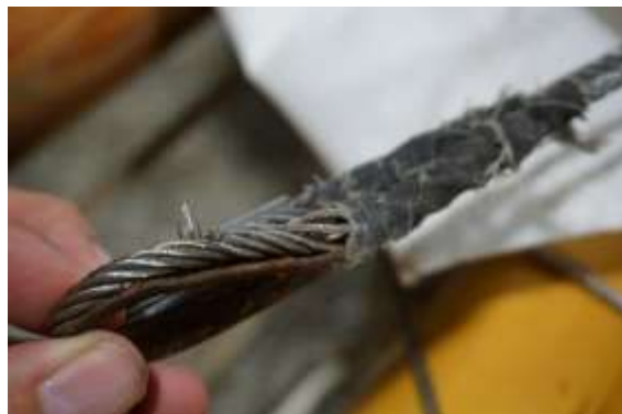
Figure 10.18 Shroud in poor condition
