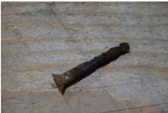
Figure 10.21 Galvanized fastener in poor condition
