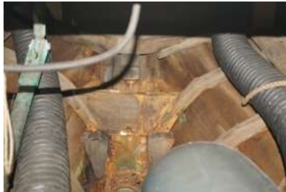
Figure 10.10 Looking aft above shaft log, note broken frames
