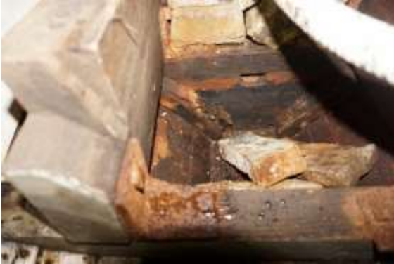
Figure 10.13 Poor frame end inboard of engine beds
